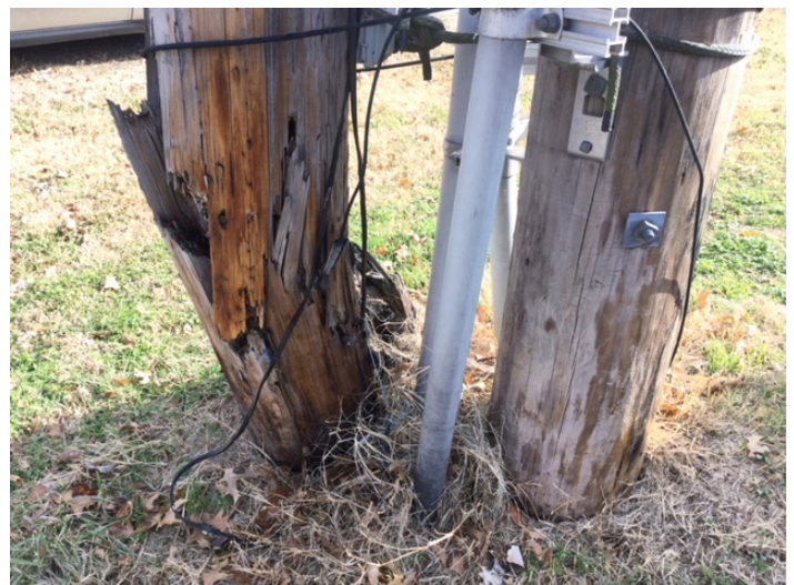
Above: Enforcement Department staff identified a broken pole in Owasso.
