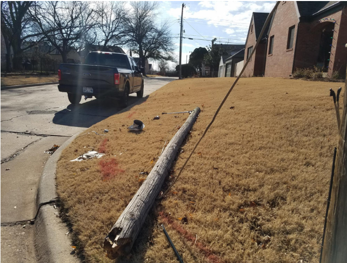
Above: Enforcement Department staff responded to a complaint of a broken pole in a resident's yard.
