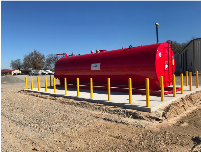
Above: An aboveground storage tank installed at Rock Haulers location. Inspection and Enforcement staff ensure new facilities are compliant with regulations.
