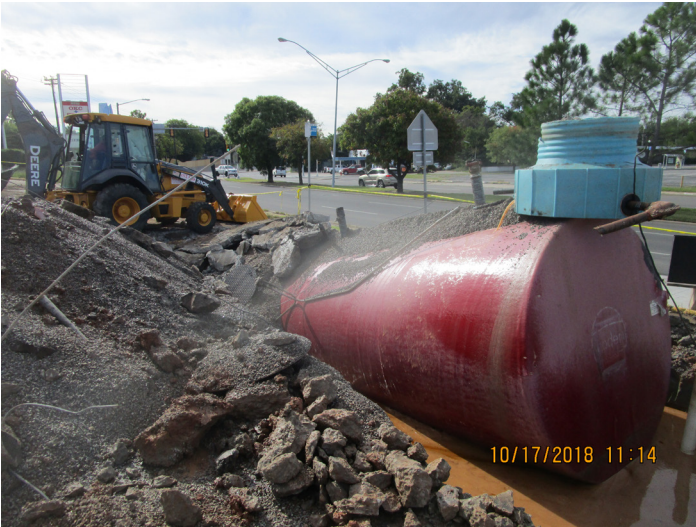
Above: An underground storage tank floated to the surface when contractors were removing the equipment. Compliance and Inspection Dept. staff oversee tank removals and issue violations if regulations aren't followed.
