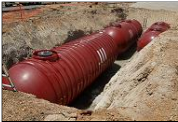
Above: Owners and operators must register their tanks with division staff within 30 days of installation .
