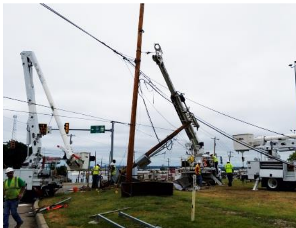
Below: PUD Enforcement Investigators assessed the damage in the Tulsa area after a tornado damaged the area in December 2017.
