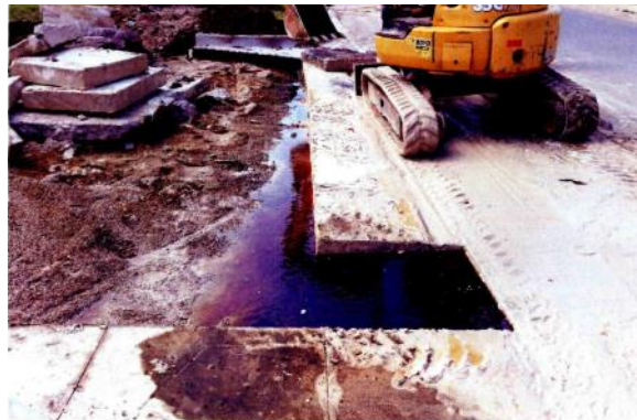
Approximately 500 gallons of gasoline leaked from a storage tank and accumulated underneath this concrete slab.
