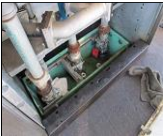
Left: Inspectors must check electrical connections at fuel dispensers to ensure the equipment is safe.
