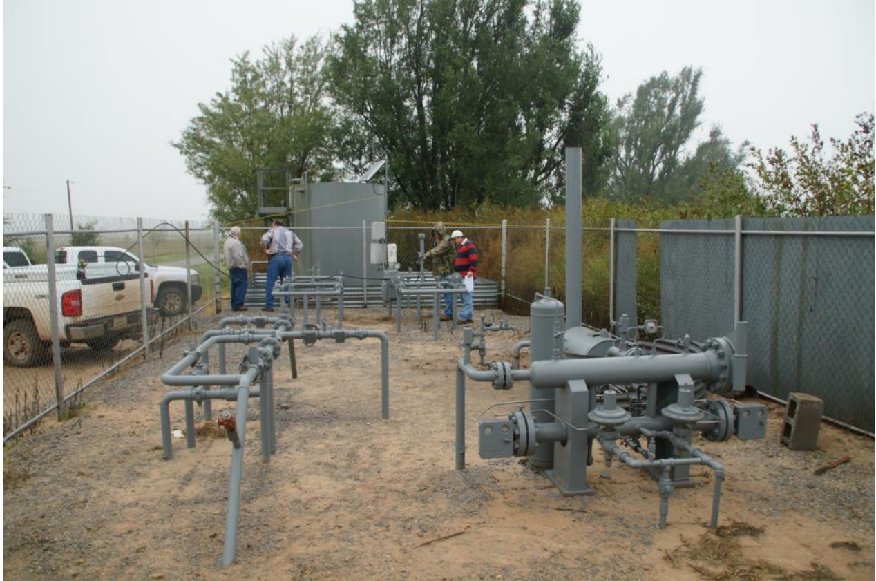
Above: Pipeline Safety Inspector Randy Kirkegard (far right) inspects natural gas relief valves at a facility in Blaine County. The Pipeline Safety Department inspects these facilities to ensure they are working correctly to protect the natural gas facilities from becoming over-pressured.
