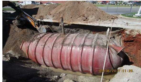
Above: The operator did not anchor this underground storage tank, which caused it to float when workers began excavation to remove it.
