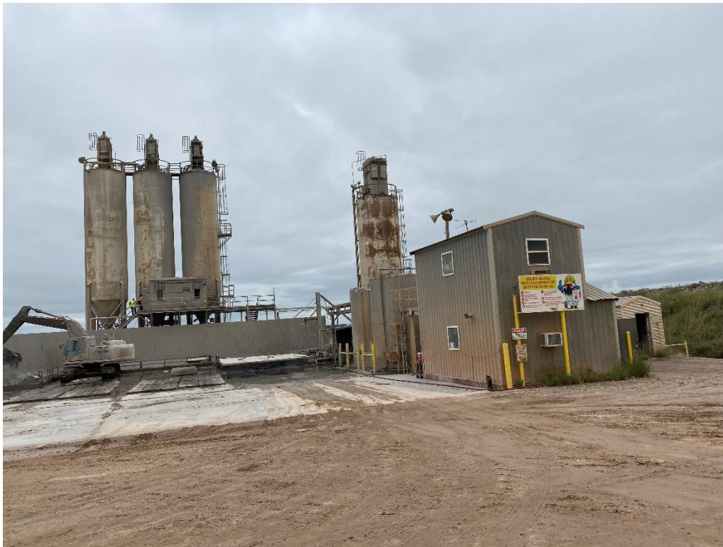
Stabilization Treatment Unit South Tank
